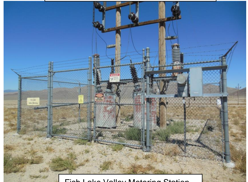
Fish Lake Valley Metering Station.
